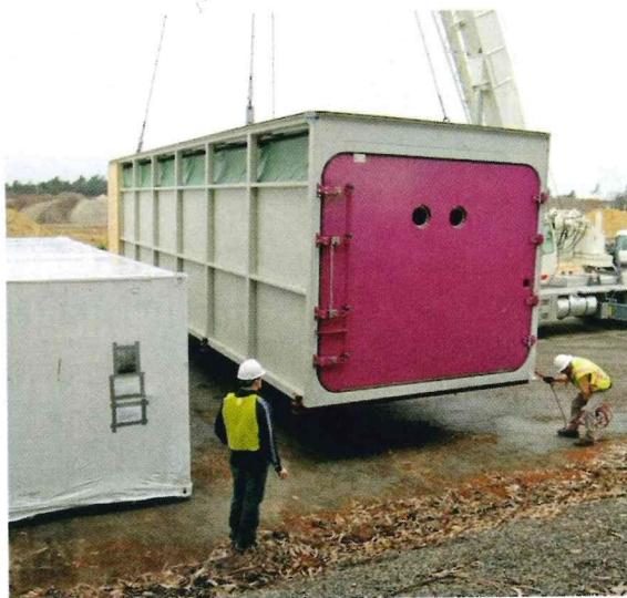
The SmartFerm containers, now manufactured in the U.S., were dropped into place using a crane.
