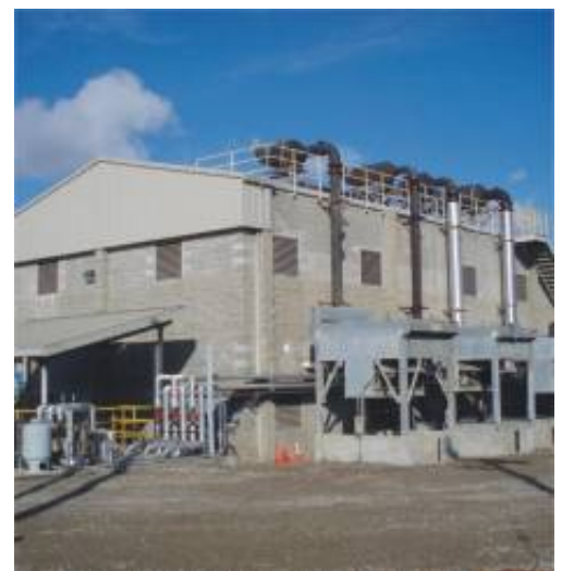
LFG building today showing waste heat recovery radiators.
