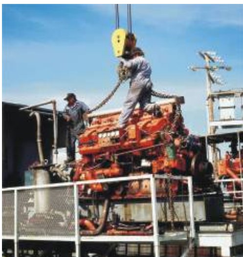
Twin trailer mounted generators were first installed in 1983.
